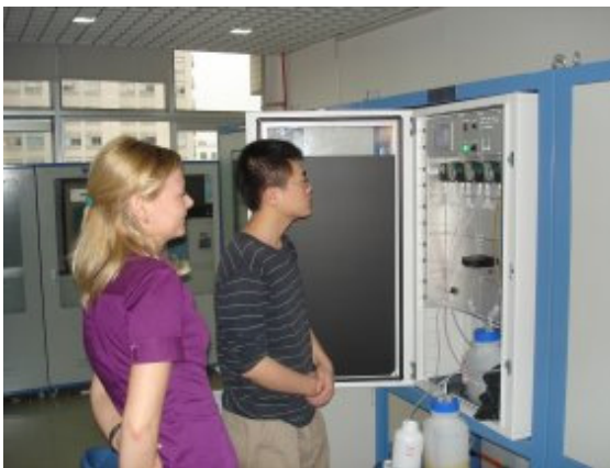
Installation in Shenzhen/China.
