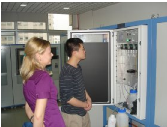
Fig. 6: Installation in Shenzhen/China.
